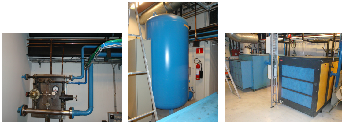
Figure D.3: Left: Pressure control panel. Middle: Buffer tank. Right: Screw compressors.
